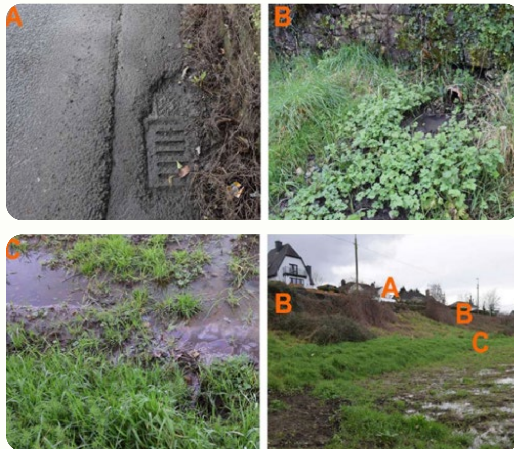
Figure 7-5: Photos illustrating the pre-existing problem at Carrick bog field: A) Road water runoff carrying silt and blocking the drains at A. B) Silt and petrochemicals are being carried into the site C) Dirty road runoff is being conveyed into the River Suir. Source: Fran Iggoe, n.d..
