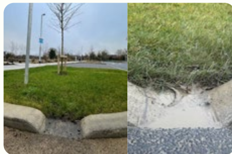
Figure 3-15: Examples highlighting situations where rain gardens were excessively filled due to a lack of understanding, hindering their ability to properly retain and filter water into the ground. Source: IGBC, 2025
